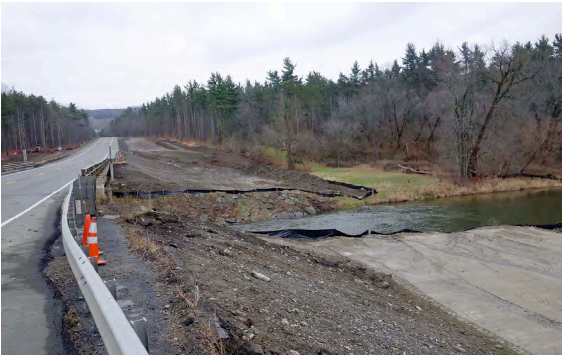
Construction area where a new highway bridge is being built across Fall Creek. The current bridge where the creek was crossed on the Cayuga Trail is on the left. See page 4 for article. Photo by Tom Reimers.
